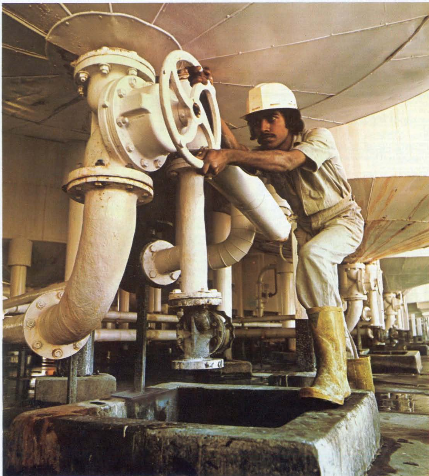
Part of the new plant for making ossein, an intermediate for gelatine, which was commissioned during 1977 in Bombay by Hindustan Lever.
